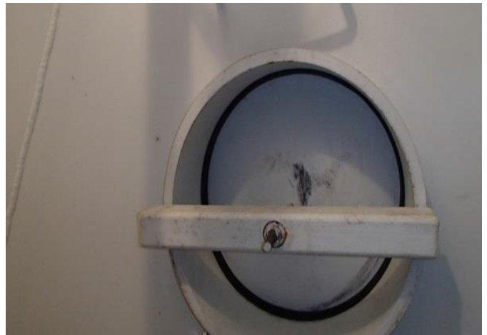
Wet Interior Boiler Manway
