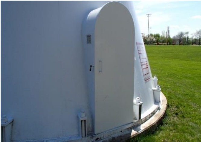
Tank access Door Locked
