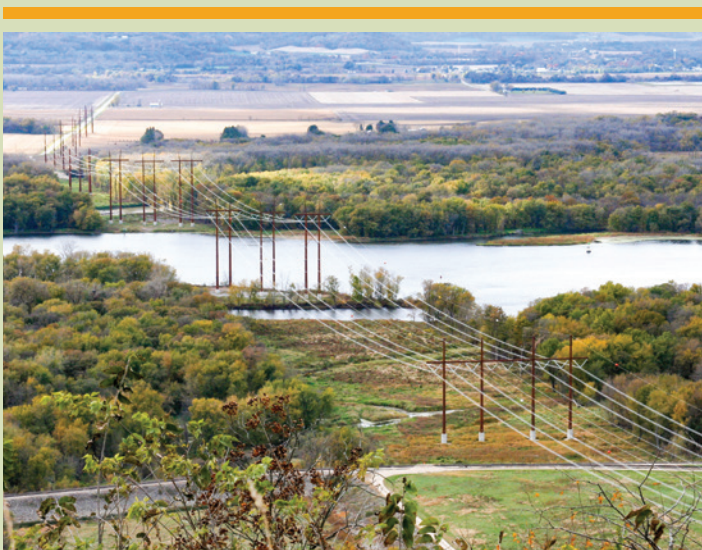
WPPI Energy owns part of the CapX2020 Hampton-Rochester-La Crosse 345-kilovolt project. Pictured is a section of the project near Alma, Wis. that crosses the Mississippi River.
