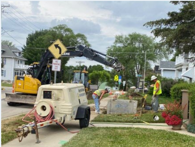
A Stoughton crew replaces a lead service line. The city successfully used directional drilling for most LSL replacements and only dug open trenches in situations where other methods were not feasible.
