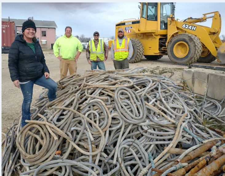
In Mayville, an impressive pile of LSLs removed. The happy crew celebrating the accomplishment includes (L to R) Courtney Steger, utilities director; Tim Gutjahr, waterworks operator; and Town and Country Underground staff Troy Hottenroth and Trevor Blake.
