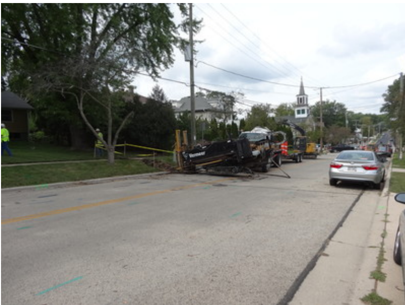
Workers replace lead service lines in Stoughton in 2021. The city has replaced all known lead lines.
