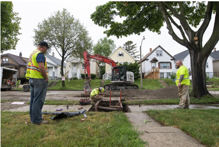
From left: Tom Iglinski, Jericho Gomez and Ryan DeBelak are part of a four-person crew working to replace a lead water service pipeline in Milwaukee on June 29, 2021. Isaac Wasserman/Wisconsin Watch
