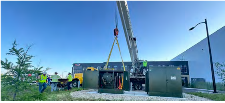
Pictured: One of three 2,000-KVA transformers being installed for a large industrial customer that recently completed their facility construction. Photo courtesy of Jill Weiss.
