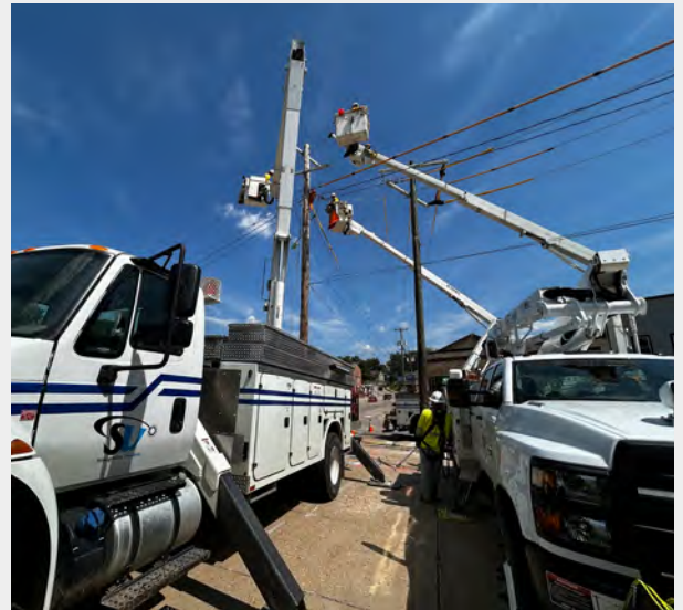
Pictured: Linemen relocating utility poles and electric lines in preparation for a DOT project on Highway 51. Photos courtesy of Andy Ruder and Scott Adler
