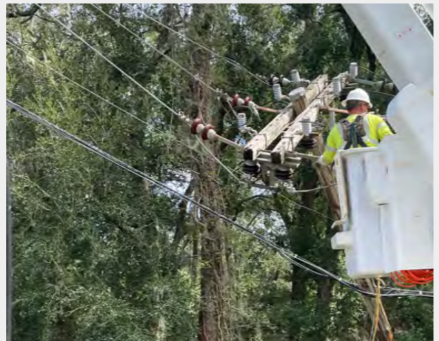
Pictured: Linecrews working to restore power to the city of Lakeland, Florida had to contend with flooding, heat, and extensive storm damage. Photo courtesy of Chad Mason.
