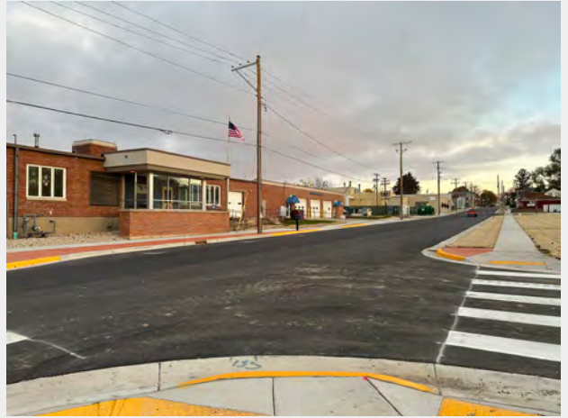
Pictured: Construction on South Fourth Street in front of the Utilities Administration Office was completed in November.
