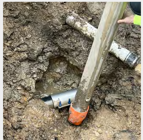
Pictured: Water main break and repair located on Van Buren Street. Photo courtesy of Dustin Kloos.
