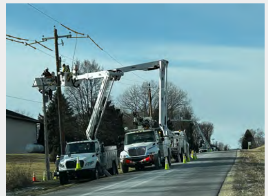
Pictured: Electric crews working on pole and line replacements on Halverson Road. Photo courtesy of Scott Adler.
