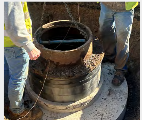
Pictured: Wastewater Operators rebuilding a manhole that collapsed on East Taft Street.
