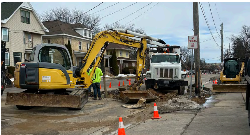
Pictured: Water Operators and contractors work to find and repair a water main break on Main Street.
